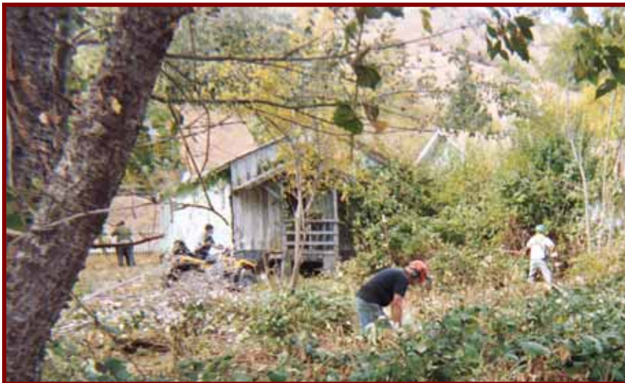
Community work day – Clearing flammable vegetation near vacant buildings in the town of Bridgeville
