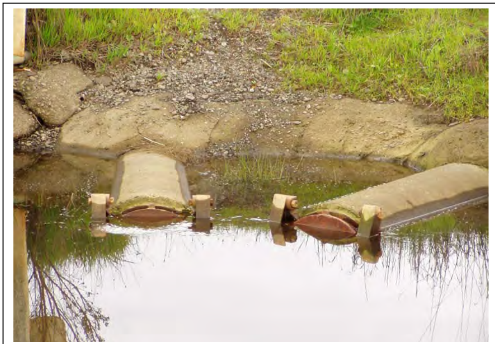
Photograph 3. Intake or outtake valves at Airport Road, camera facing northeast. .
