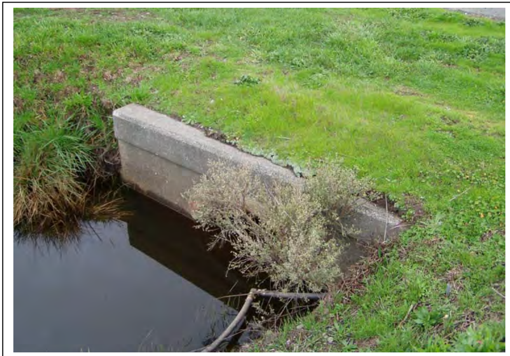
Photograph 4. Outtake valve on the south side of Airport Road, camera facing southwest.
