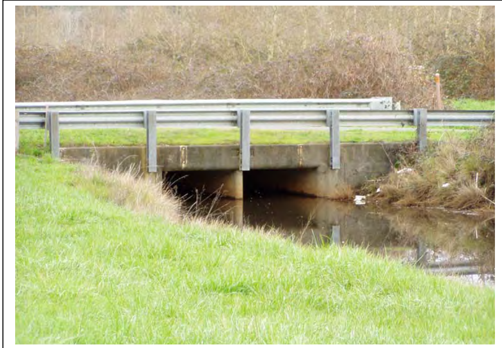
Photograph 5. Culvert located across from Arcata Lumber mill north entrance, camera facing northeast.
