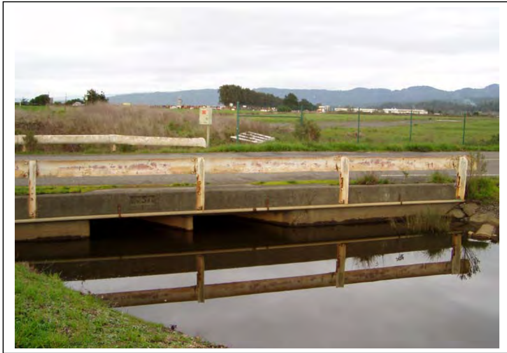
Photograph 2. Culvert at Airport Road carrying the road over the ditch, camera facing northwest.
