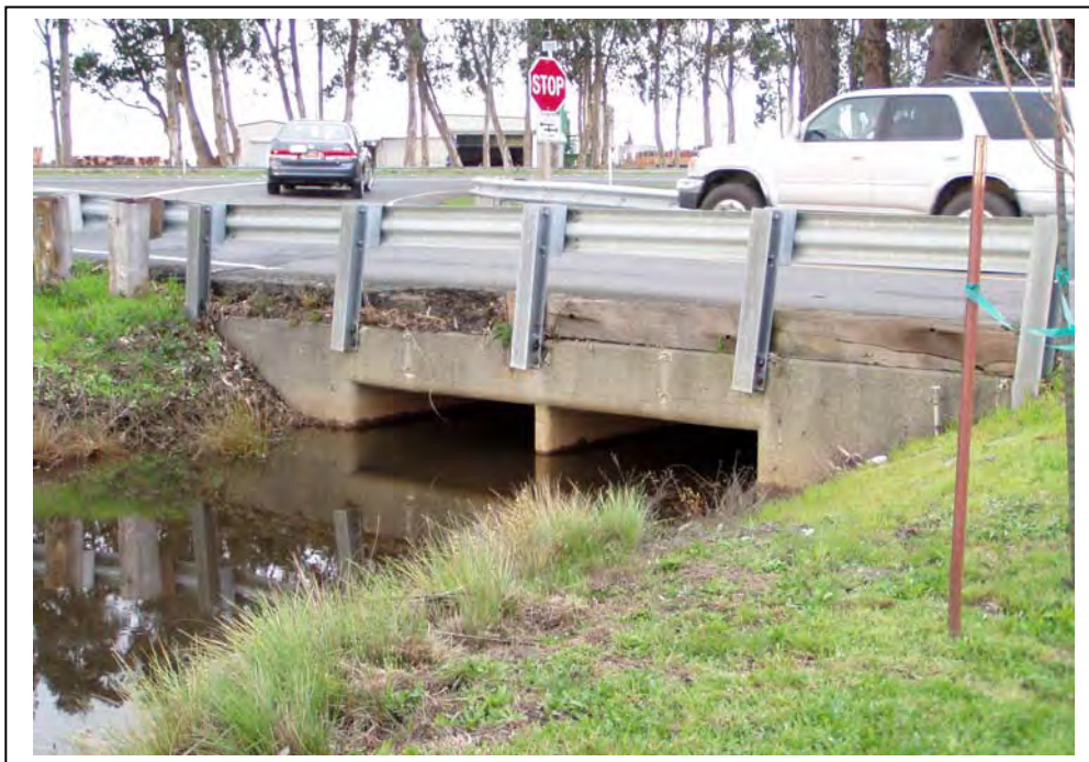
Photograph 5. Culvert located ½ mile north of Airport Road at the Toyota Dealership, camera facing northwest.
